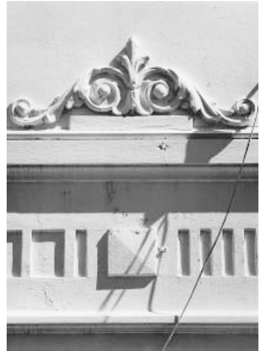
Detail, Randolph Street, Pump No.11
