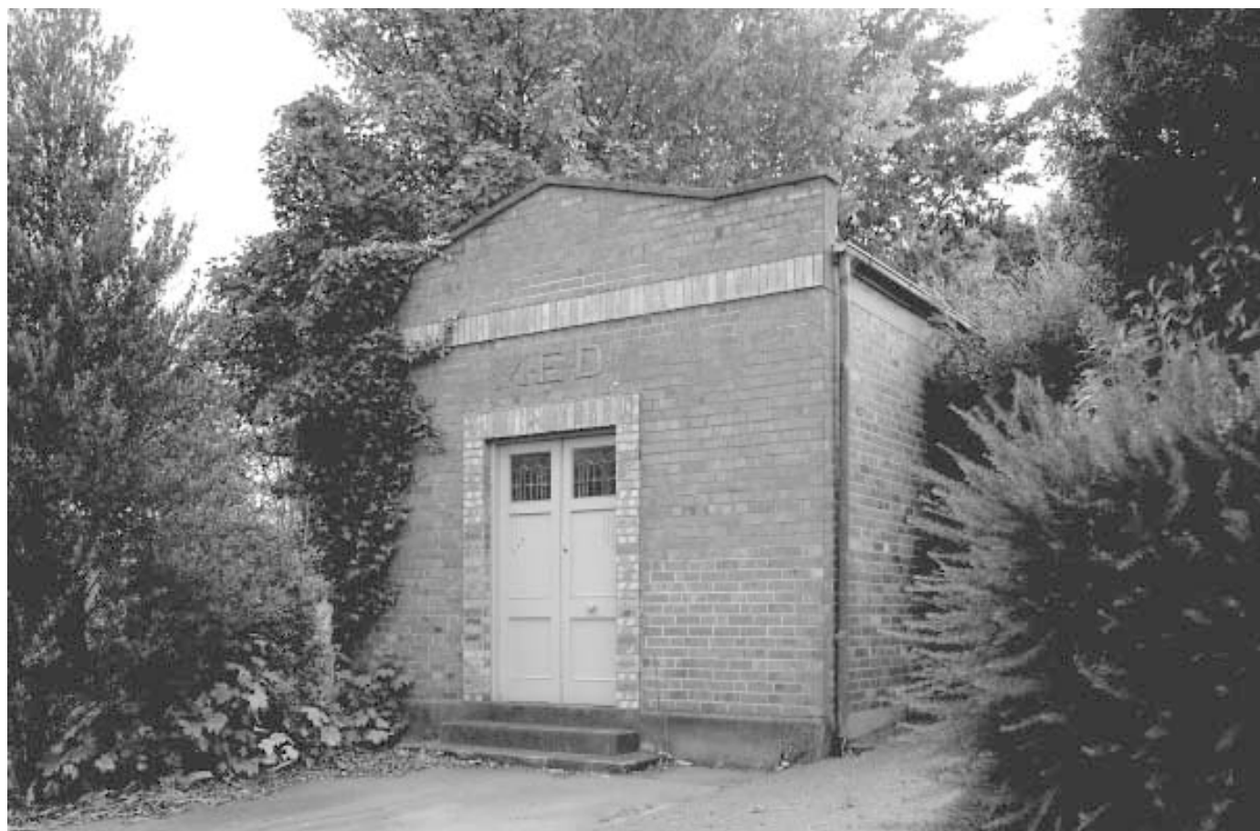
Office Road West Substation
