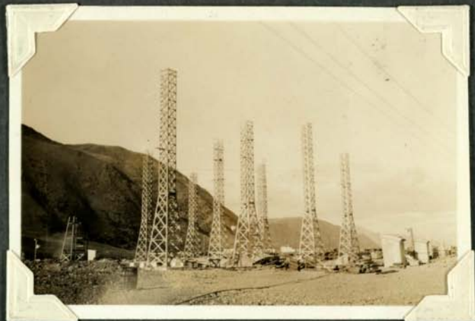
Outdoor Station steelwork. Towers 50 FT & 43 FT High.
