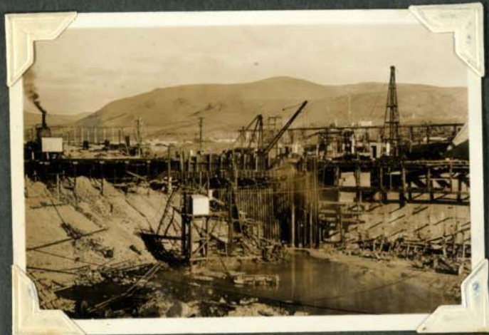
Excavation in Cofferdam Sheet piling partly removed. Outdoor station steel towers in background on left.
