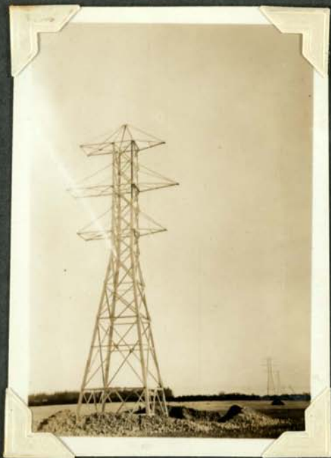
Start of line showing terminal strain tower 40FT. 45FT. suspension towers in background.
