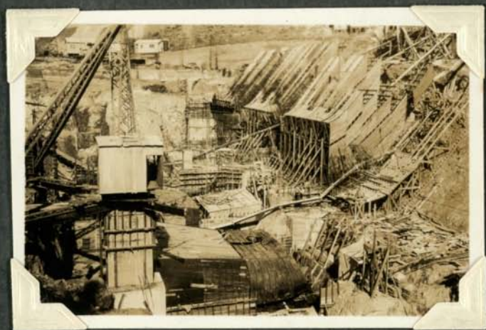
Powerhouse. Steel liner of No 2 Draft tube being fitted in position. Penstock forms for No 3, 4 + 5 units in position.
