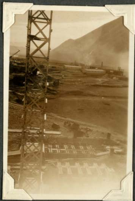
Outdoor Station. View from top of tower K. O.C.B. pads & pad for tower C just completed. Dam in background.
