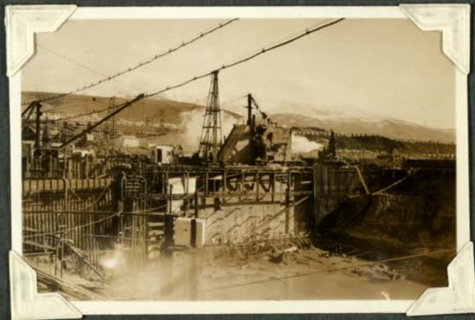
Cofferdam. Cut off wall excavation on right. Village houses in background. Drag-line excavator tipping into hopper
